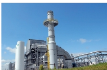
Net-Zero Hydrogen Energy Complex to Supply Low-Carbon Hydrogen for Production of Renewable Diesel in Canada
