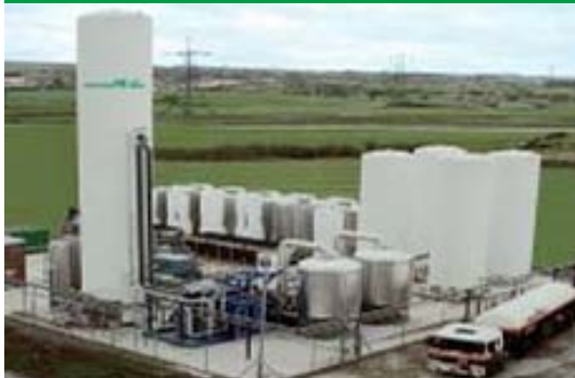
Onsite Gas Supply
