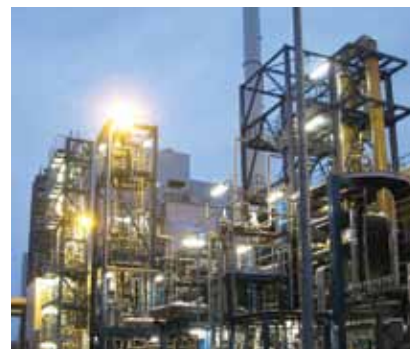
Air Products’ CO 2 purification unit at Vattenfall AB’s Schwarze Pumpe, Germany, oxyfuel pilot plant facility.
